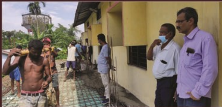
Work in progress: Roof casting of the ongoing construction of Late Geetarth Barua Memorial Library Reading Hall cum Exhibition Centre.
